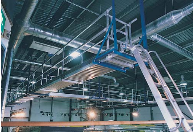
The permanent installation of a suspended Spandeck walkway in the Royal Signals Museum provides access to roof work areas such as air conditioning without closing exhibition to the public.
