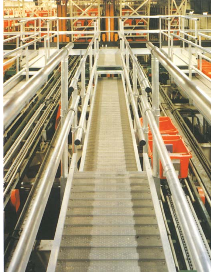
John Lewis Partnership - Access to stock picking conveyor system in warehouse.
